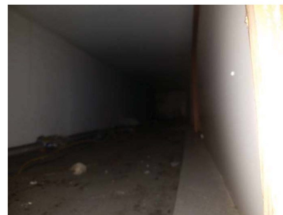
INACCESSIBLE OVERHEAD STORAGE AREA IN PLAYMATES
